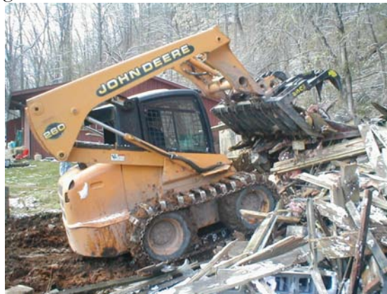
Cavers got some mechanical assistance in removing the remains of the Octagon House at Grand Caverns during the Easter Restoration Field Camp. (Photo by Jim McConkey)
